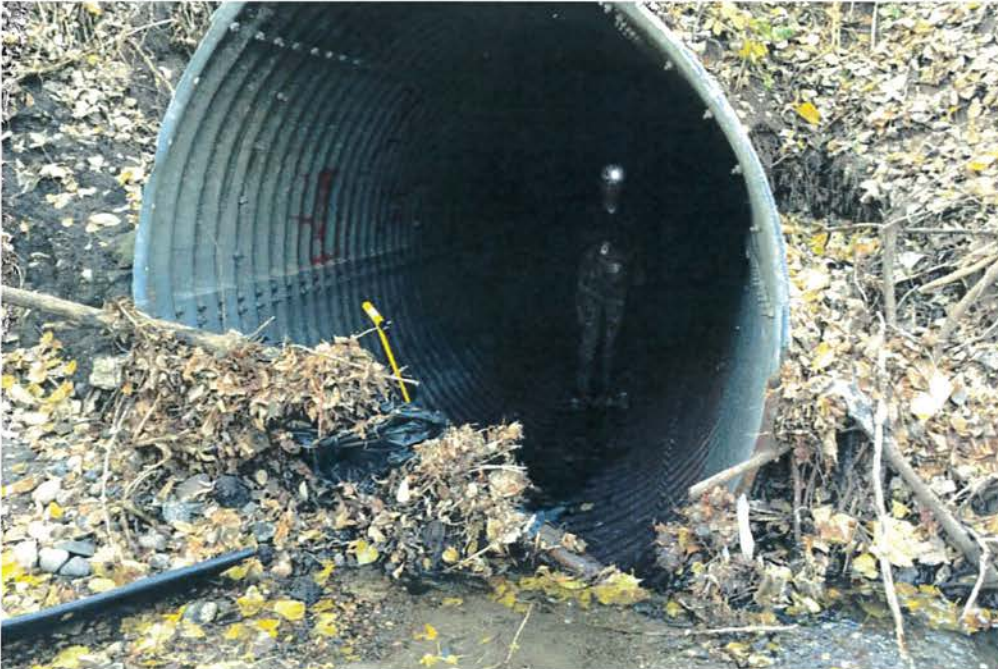
Figure 4-3 Sediment and Debris Accumulation at the Culvert Inlet
