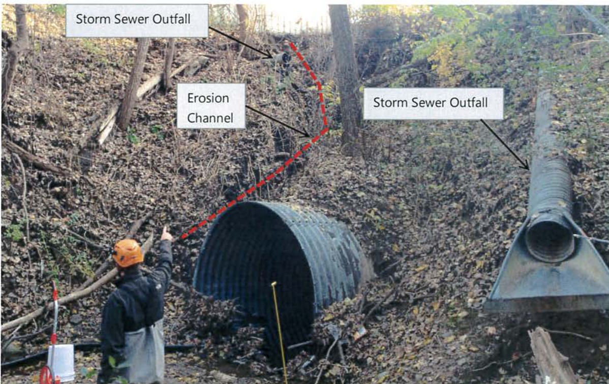
Figure 4-1 Existing Erosion and Storm Drain Outfalls at the Culvert Inlet
