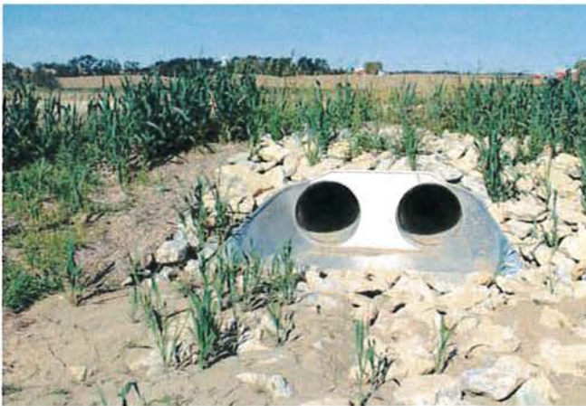
Figure 5-3 Metal Inlet Structure
