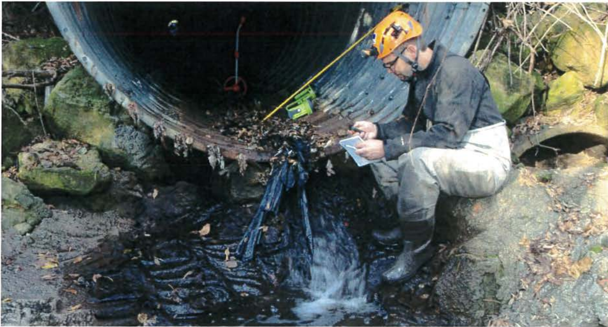
Figure 4-4 Base Flow Traveling Outside of Culvert at the Culvert Outlet
