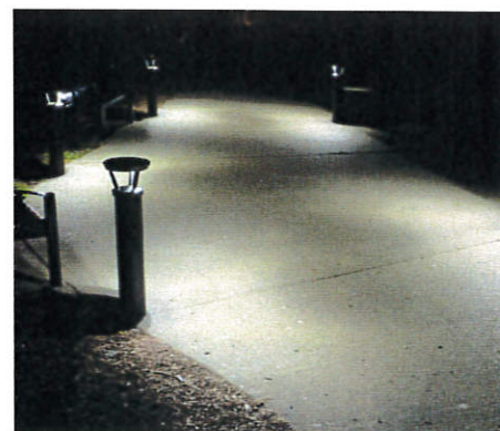
Example of pedestrian-scaled path lighting designed to illuminate the path only
