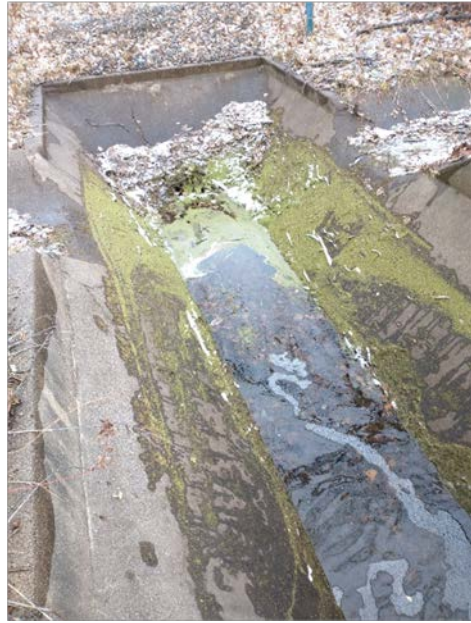
T-8 Pond pipe inlet (partly blocked)
