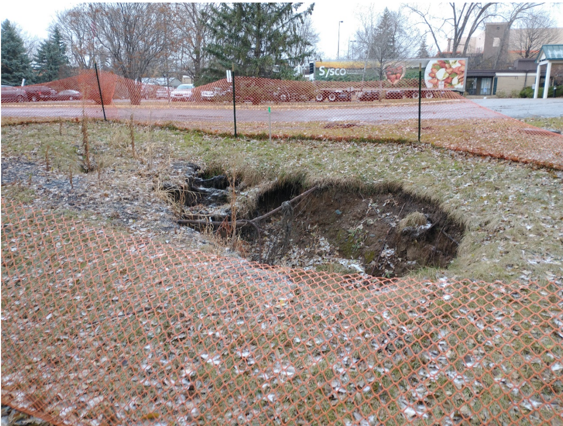
Sinkhole above storm sewer pipe, near southeast corner of upper parking lot
