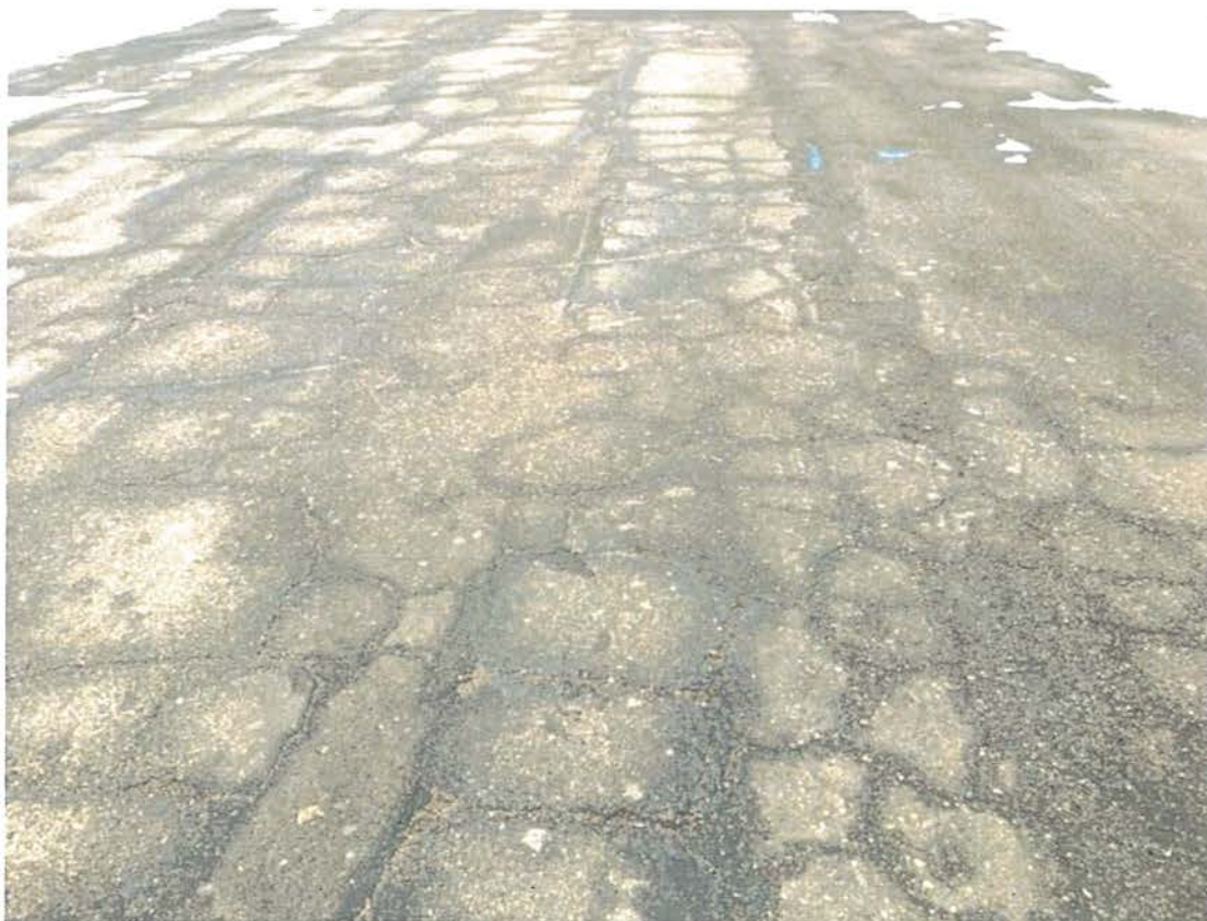
Figure 4. Typical patching, block cracking, severe longitudinal cracking, and raveling on 55 th Court.
