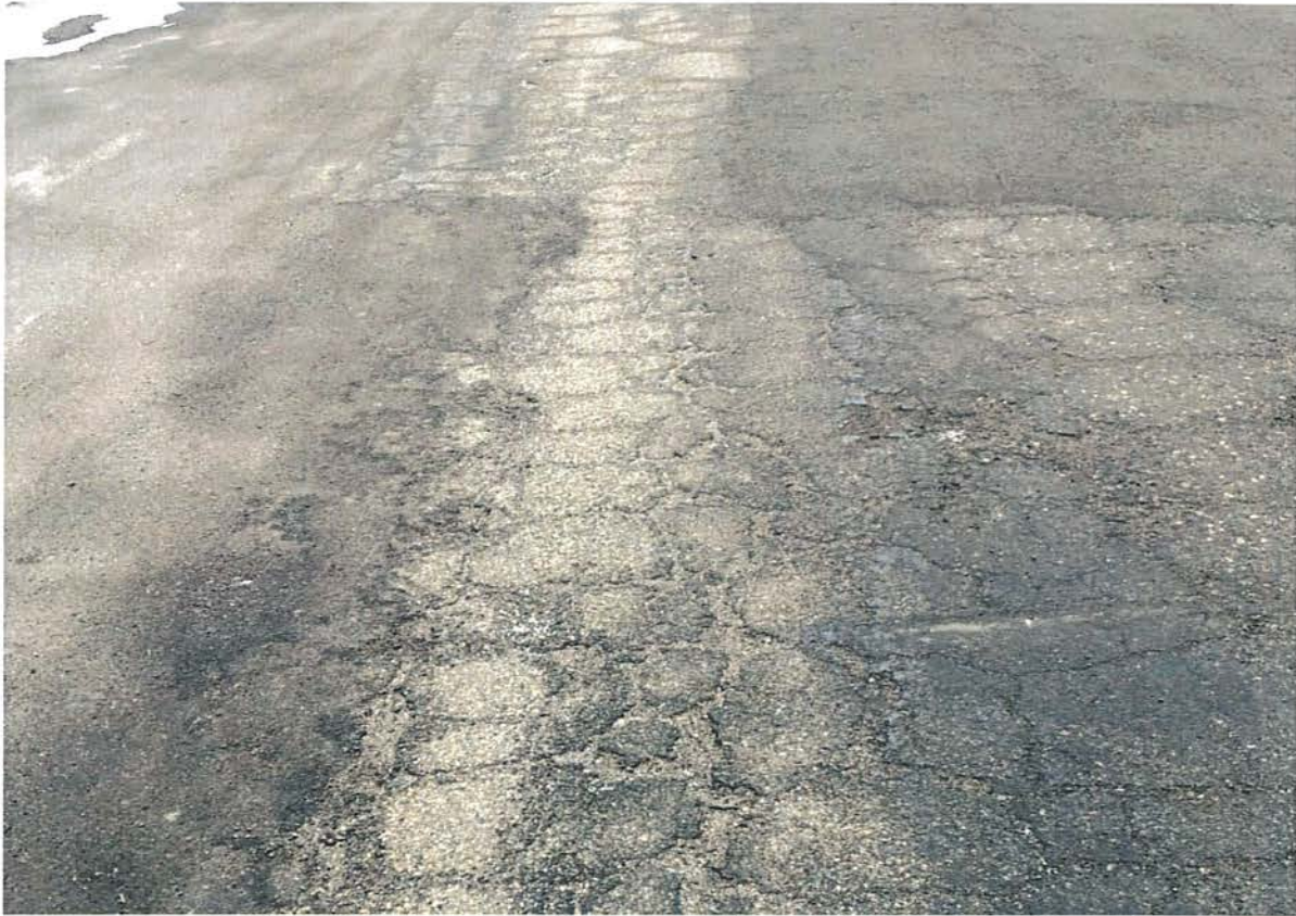
Figure 2. Typical skin patching, fatigue cracking, raveling, and possible rutting.
