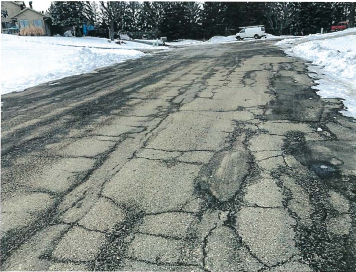
Figure 1. Typical patching, severe longitudinal cracking, raveling, block cracking, and rutting.
