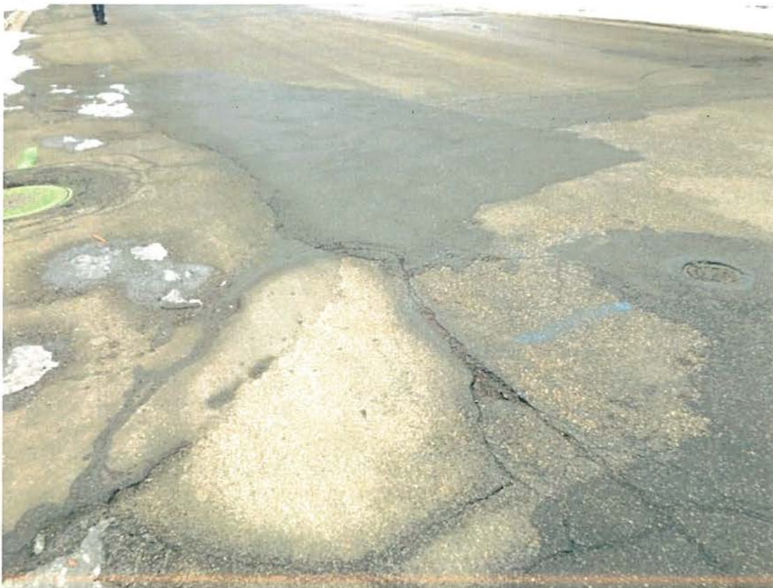
Figure 3. Typical patching, severe longitudinal cracking, raveling, and block cracking on 55 th Street.
