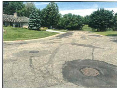
Existing Pavement Condition
